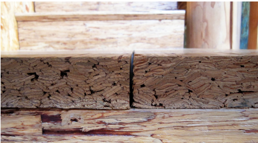
Figure 18: The raw edges of the recycled, FSC-wood stair treads at IslandWood are left exposed, eliminating the need for finish materials.
