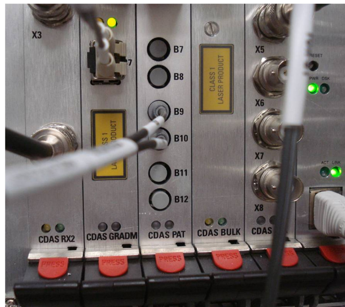
Figure 1.59. Connection to CDAS (picture from Phillips)
