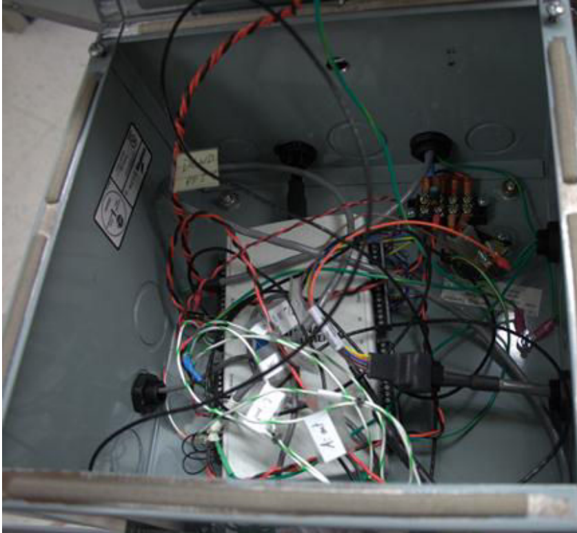
Figure 1.8. View of DAQ and wiring inside of the smaller project box
