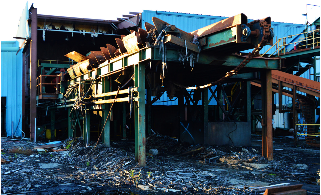
Fig 2.17: Remnants of the debarking station at the Beaver Division of the Interfor Mill.
