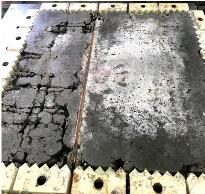
Figure A.6: Panel with poor consolidation
