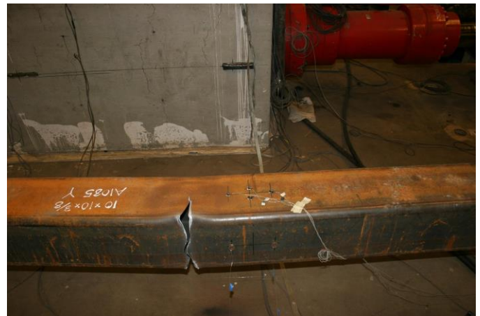
Tearing Across East Wall: 1.75" Cycle 2 T
