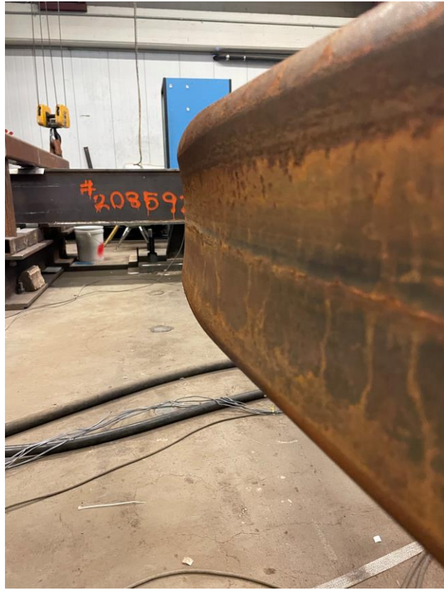
'Kaldestad effect' on outside face of brace while buckling
