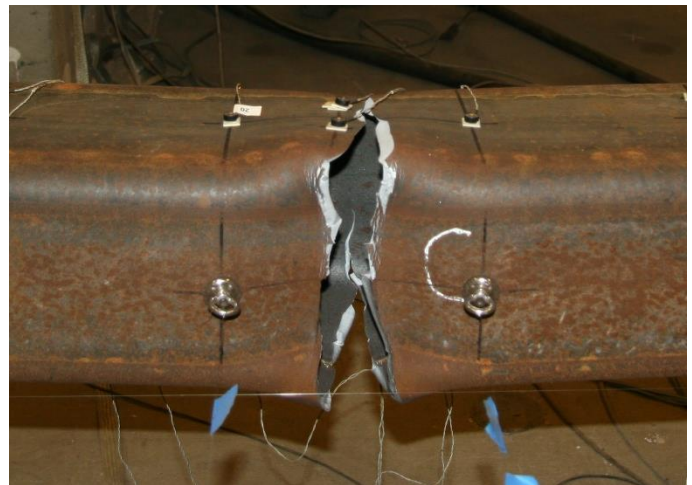
Brace tearing at incipient fracture: cycle 19
