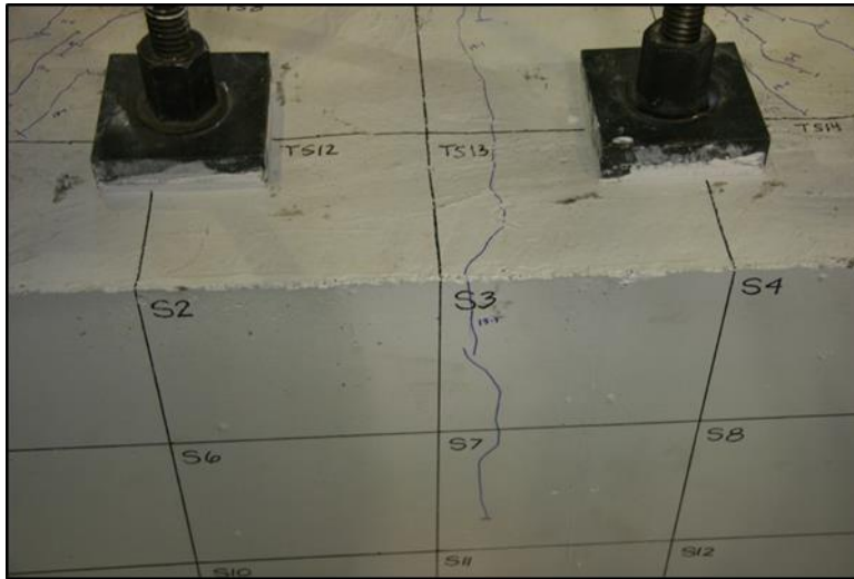
Figure 5.24: WRC cracking on South face of cap beam at 7.04% drift
