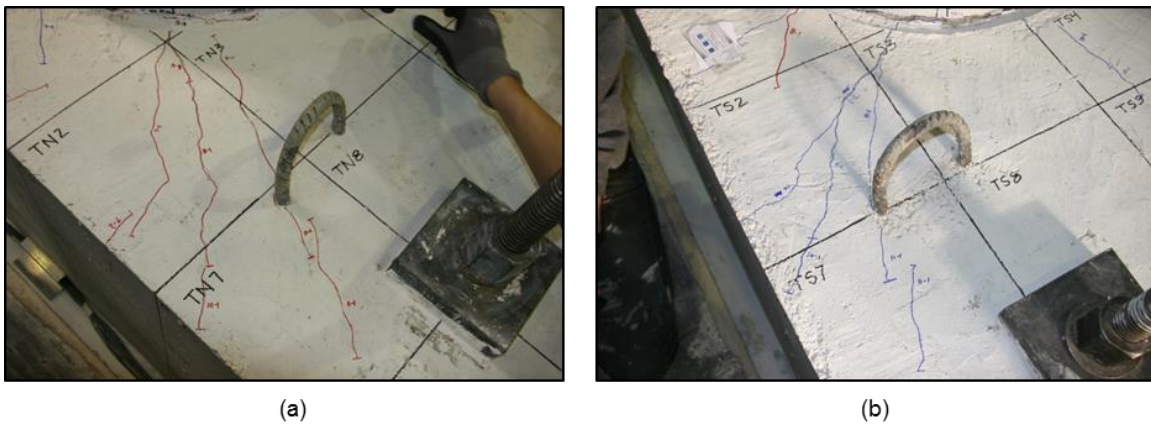
Figure 5.23: WRC cap beam cracking during the 11 th cycle level (a) North side of specimen, (b) South side of specimen
