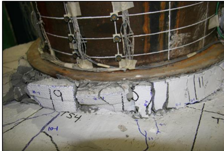
Figure 5.34: WRC South soffit damage at 11.47% drift South
