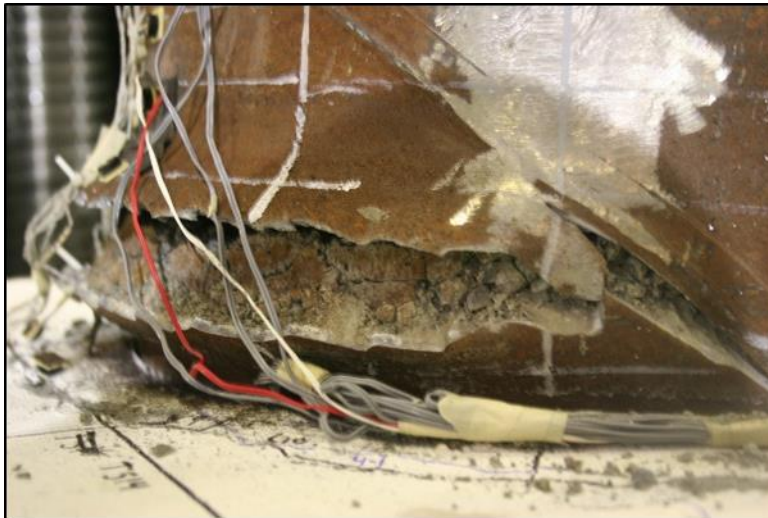
Figure 5.13: EMB80 tear propagation on South side of column at 8.30% drift
