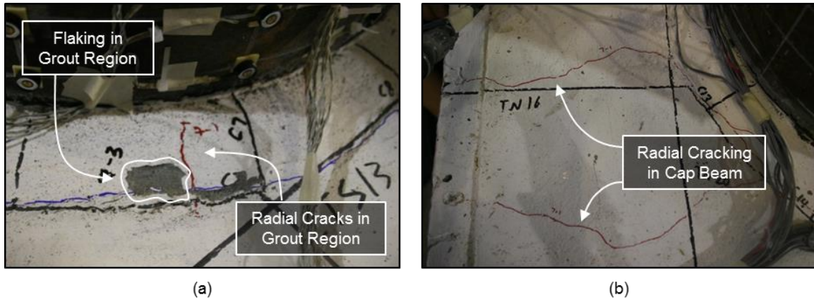
Figure 5.6: EMB80 Radial cracking at 1.45% drift in (a) grout region, and (b) cap beam
