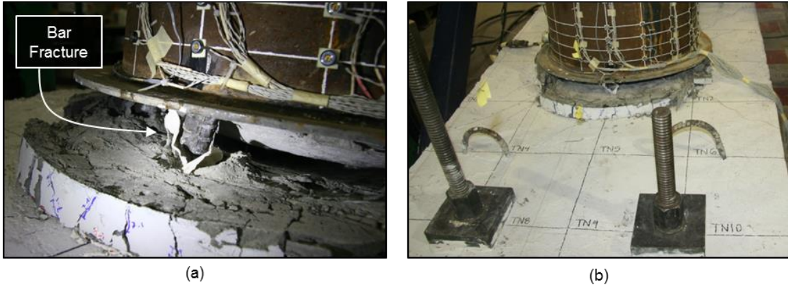
Figure 5.48: WRCUB (a) North bar fracture, and (b) North cap beam damage at 12.27% drift South
