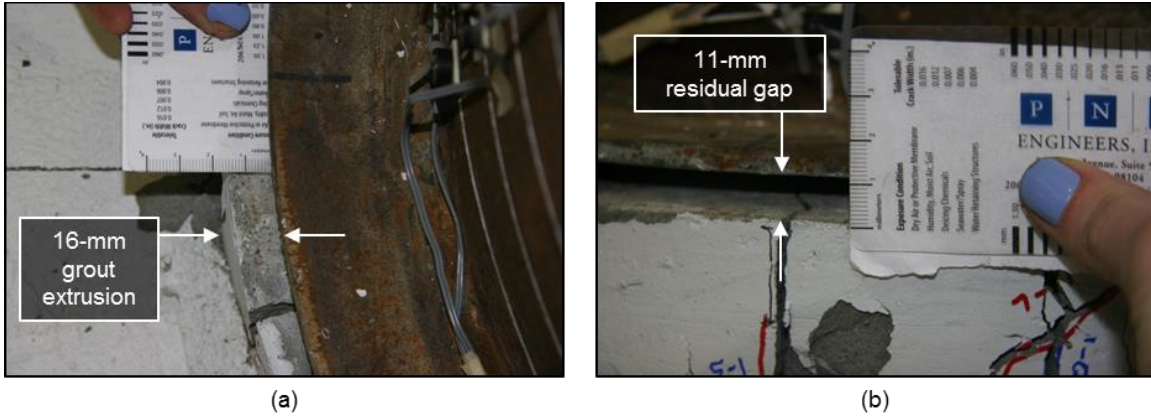
Figure 5.44: WRCUB (a) grout extrusion, and (b) residual soffit-flange opening after 13th cycle level
