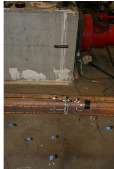
Brace Tearing: 4.75" Cycle 1
