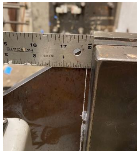
Figure 4.3. Measured Bolt Slip at South Gusset Plate
