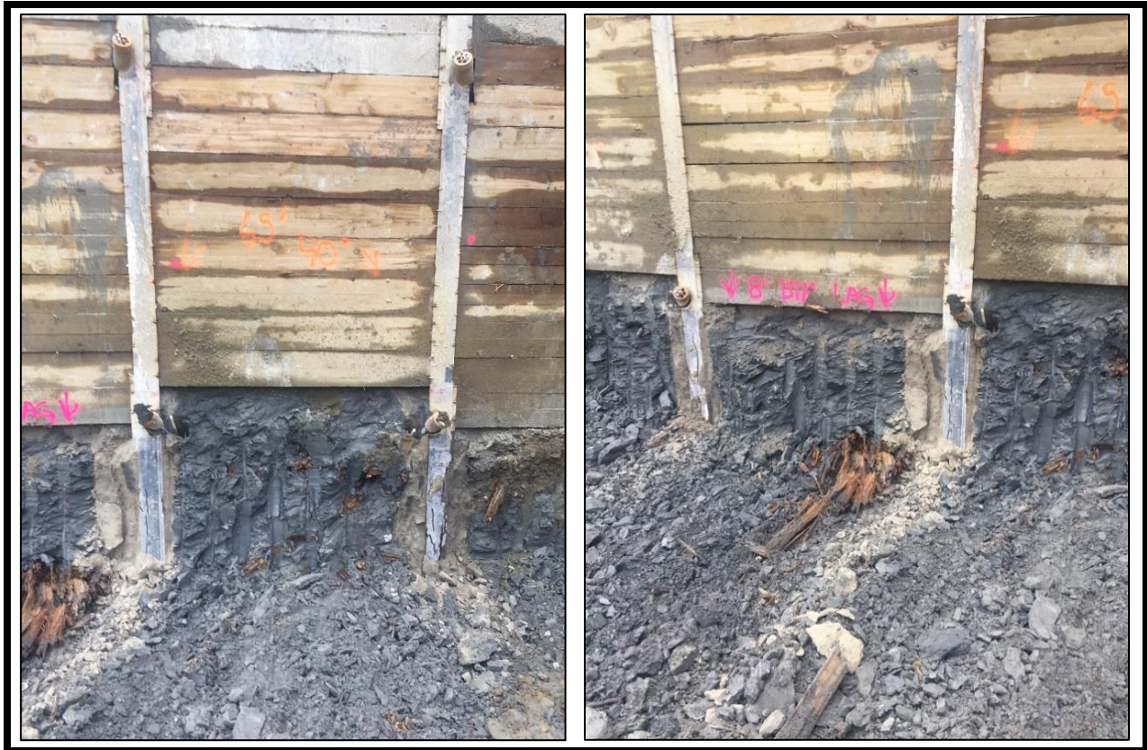
Figure 7. Site Recon Photos: Photographs taken at the excavation at 8 th and Thomas, Seattle, Washington, on February 14 th , 2017. Sediment layer below the lagging (wood crib wall) is Qob, as evidenced by the grey sandy silt and prominent wood. The bottom of the excavation is approximately 44 feet below ground surface. The wooden planks shown in the photograph are 12 inches in from top to bottom.
