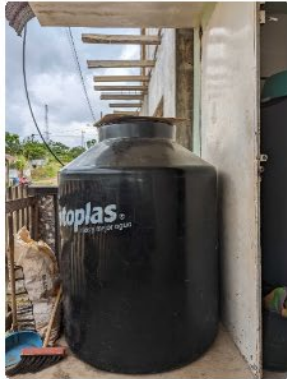
Large water tank (outside)
