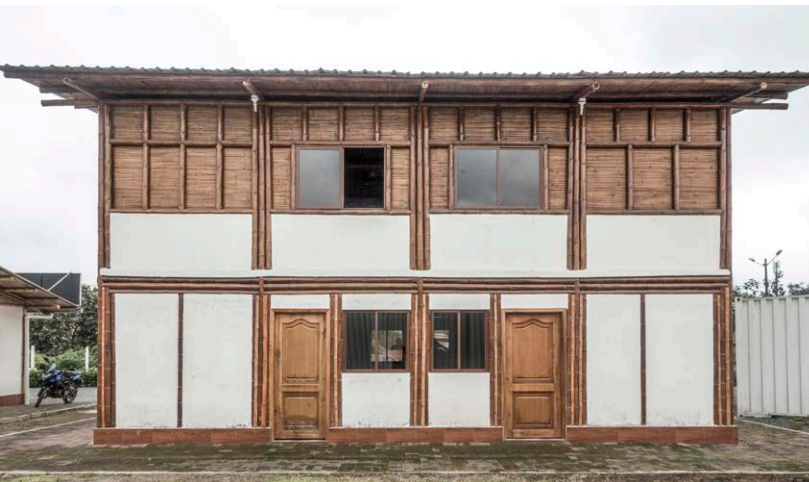
Fig B.76 - Two story prototype showing weathering issues only a few years after built, Santo Domingo, Ecuador
