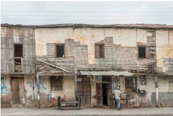
Fig 5.34 - Homes in disrepair. Bahia de Caraquez, Ecuador
