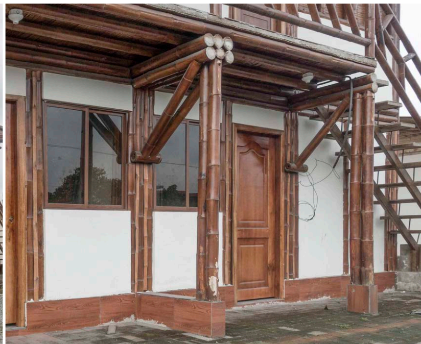
Fig B.79 - Two story prototype showing weathering issues only a few years after built, Santo Domingo, Ecuador
