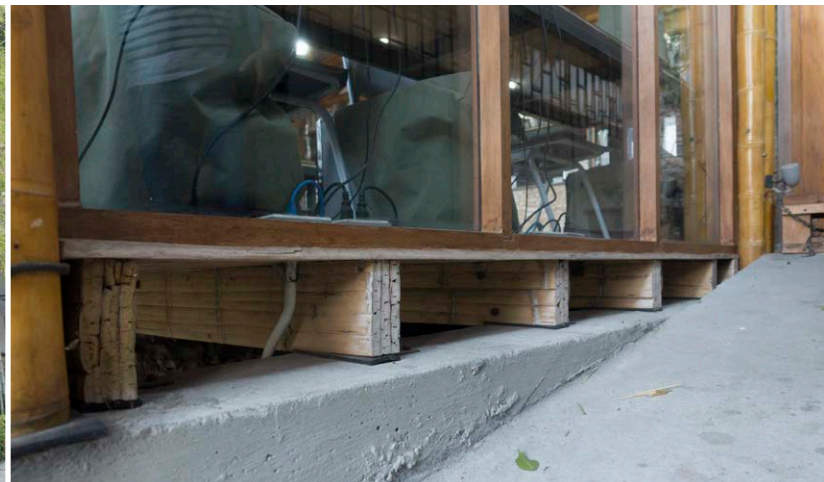
Fig B.3 - Innovative glue-lam bamboo floor joists Bamboo Library, Catholic University of Guayaquil, Ecuador
