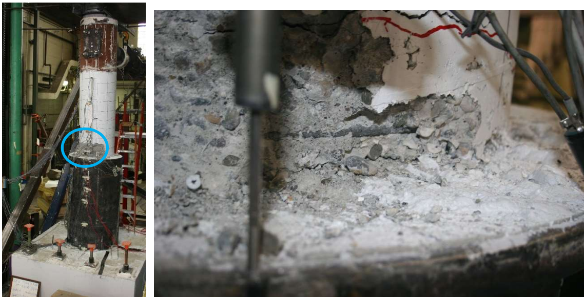
Figure 4.79. Specimen 30-21-R Exposed Transverse Reinforcement at 4.0% Drift
