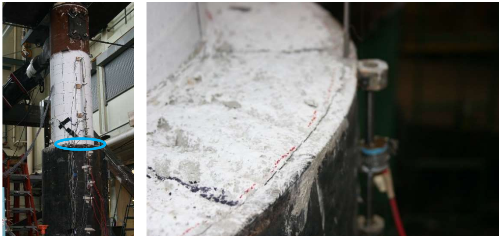
Figure 4.98. Specimen 30-21-LD Cracks at Edge of the Pile at 0.7% Drift
