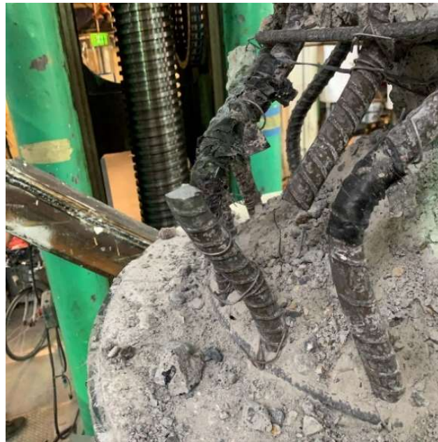
Figure 4.92. Specimen 30-21-R Fractured Longitudinal Reinforcement
