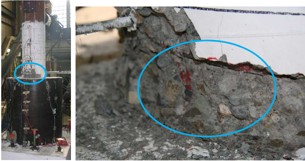
Figure 4.51. Specimen 48-21 Exposed Transverse and Longitudinal Reinforcement at 4.1% Drift
