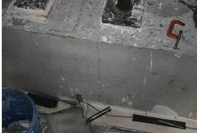
Figure 4.113. Specimen 30-21-LD Crack on Southern Side of Transfer Block
